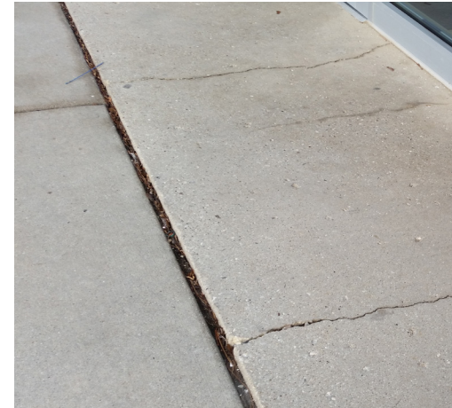
Exit landing cracks
