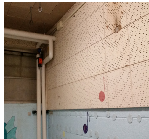
Stained ceiling and wall tiles
