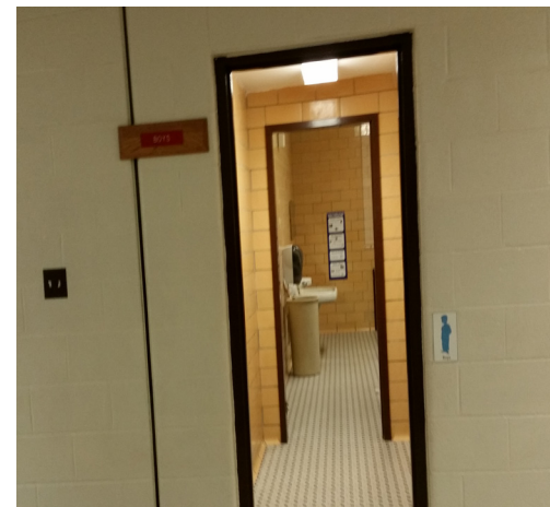
Narrowed door frame passages
