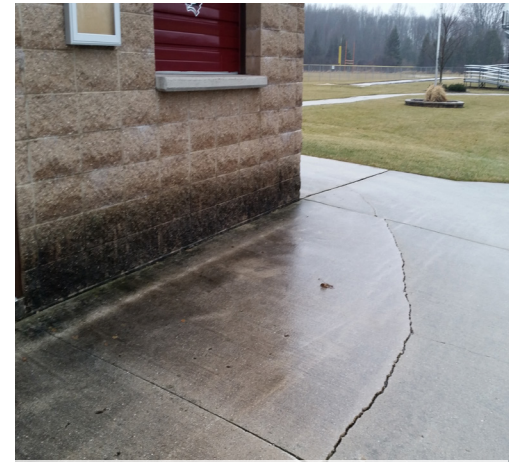
Existing walking cracks
