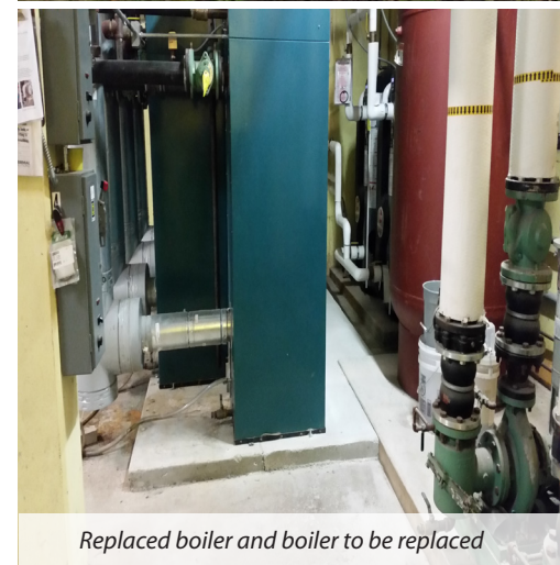
Small zone air conditioning units
