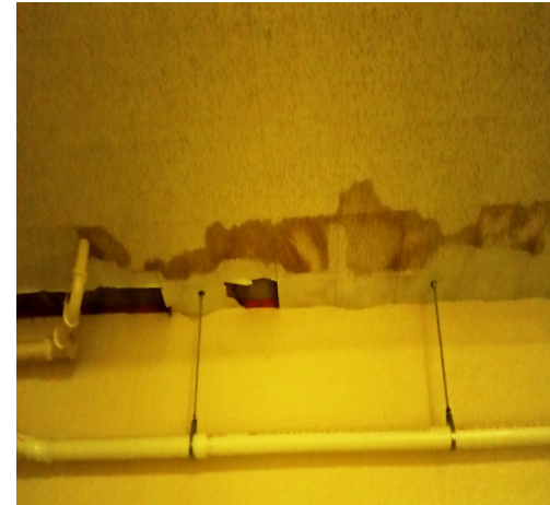
Open wall and ceiling penetrations
