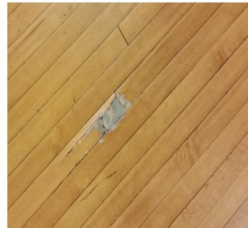
Damaged wood gym floor
