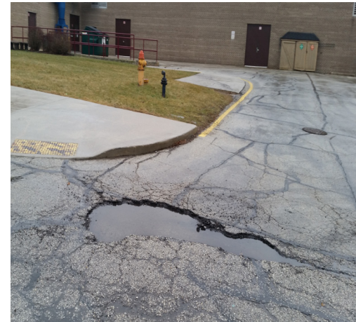
West lot asphalt pot hole
