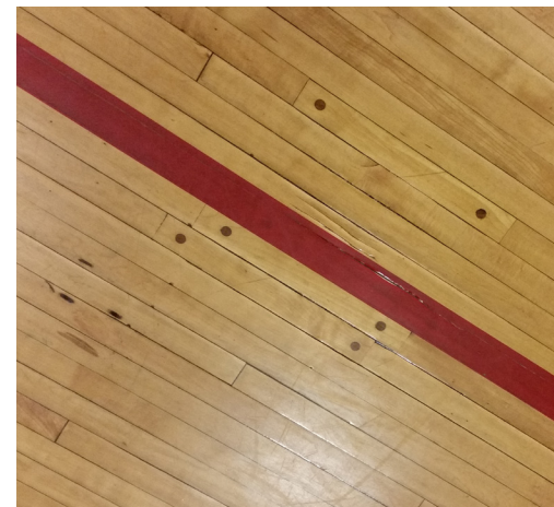
Damaged wood gym floor
