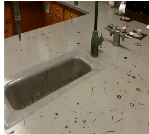
Damaged work table
