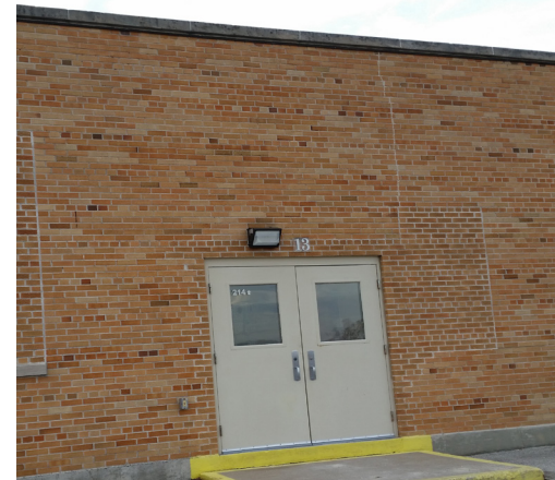
Gaps along building perimeter
