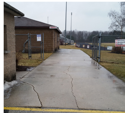
Existing walkway cracks
