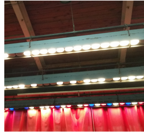
Stage lights and suspension system
