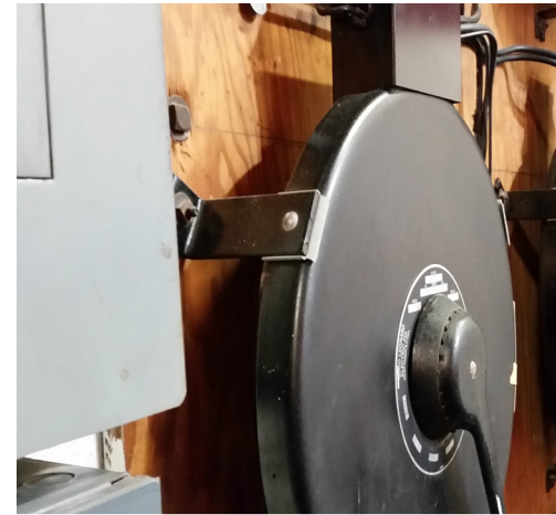
Stage electrical panels and dimmers
