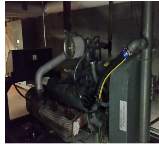
Old high school generator
