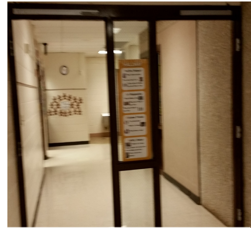
Missing corridor separation doors
