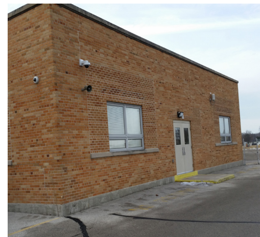
Gaps around building perimeter
